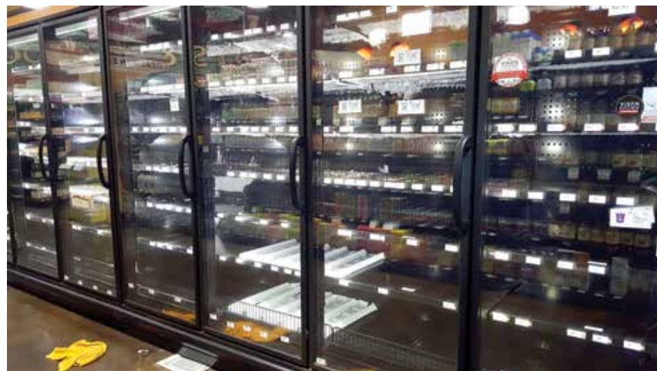
Bare shelves in the frozen department of North Coast Co-op's Eureka store during the refrigeration and freezer system failure.
